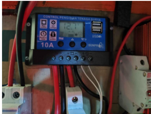
Figure 15. SCC display indicating a fully charged battery (12.7V)
