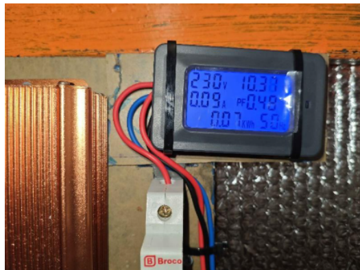
Figure 16. Wattmeter reading during normal system operation
